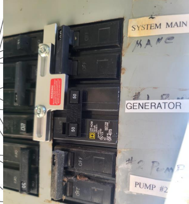
Emergency power transfer switch
